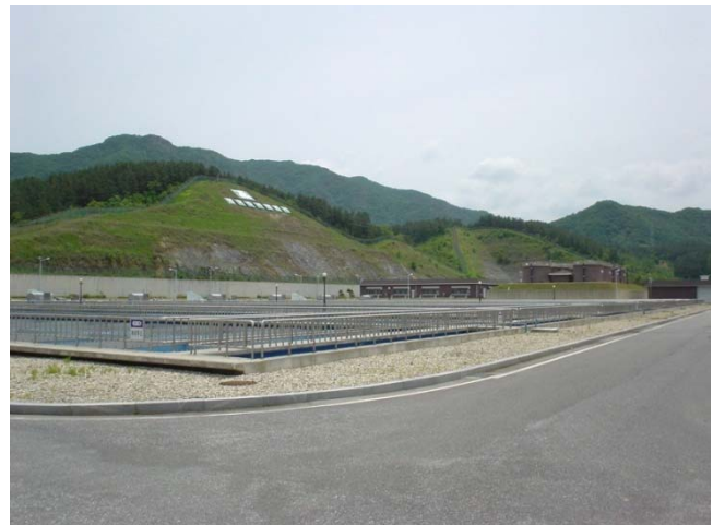
Sedimentation basins in Gosan. One of five production plants at the Southern Geum River Water Supply.
